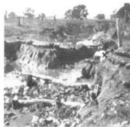
ROAD BADLY DAMAGED. The Appila-Tarowie main road at Fetherstonhaugh's Creek, showing the serious damage done by the recent floods in the North. The stones mark the centre of the roadway. Traffic had to be diverted.
